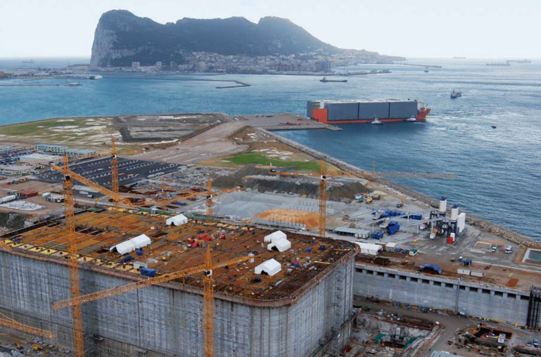
The gravity-based offshore structure for the Adriatic LNG terminal (foreground) is as long as four football fields and as tall as the Statue of Liberty. Its two large storage tanks will hold enough LNG to generate a month's worth of electricity for about 1 million homes in northern Italy.
