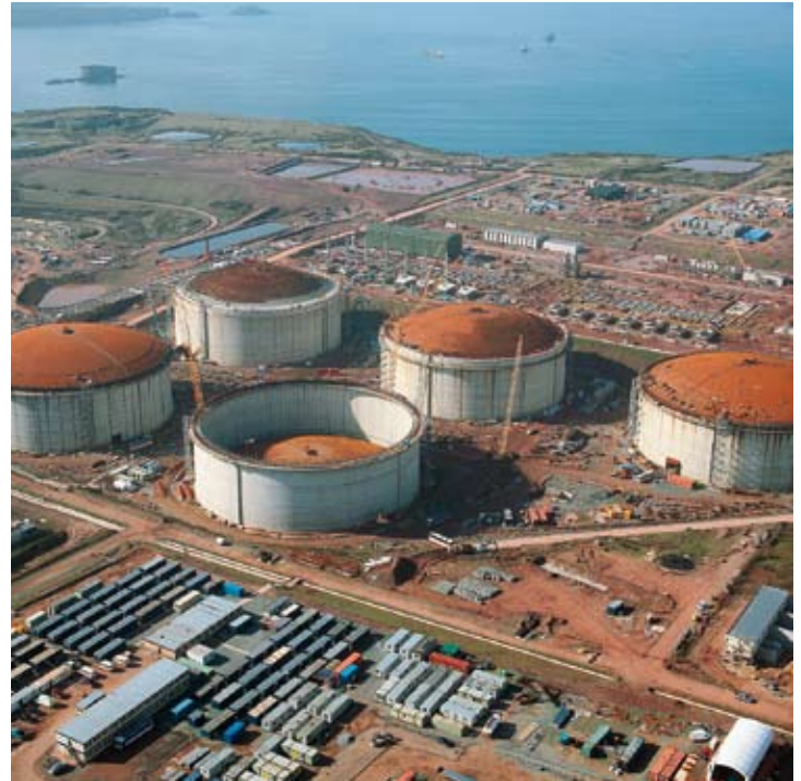
The South Hook Terminal in the U.K. is being built on the site of a former Esso refinery.
